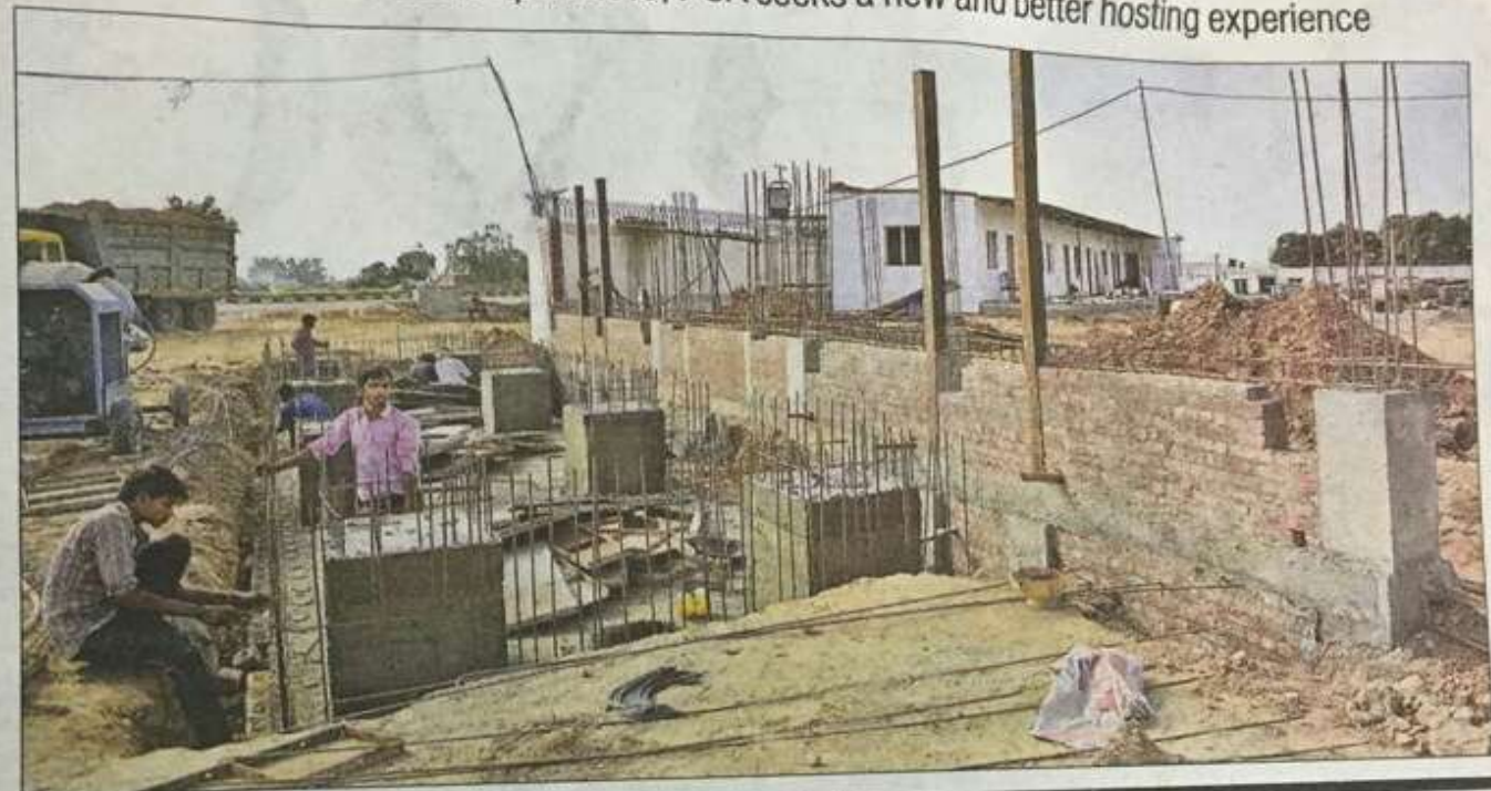
Work in progress at the site of the new stadium of Punjab Cricket Association on the outskirts of Chandigarh. RAVI KUMAR/HT
